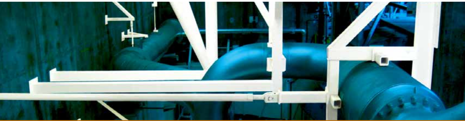
Seismic bracing inside Columbia
